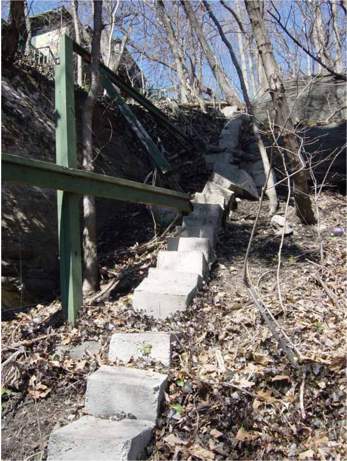
Figure 3: Slope processes at Harpers Ferry. Slope creep and erosional undercutting have undermined this private stairway above Harpers Ferry National Historical Park. Such processes have the potential to destroy trails along slopes and bury features below. Photograph by Trista L. Thornberry-Ehrlich (Colorado State University).
