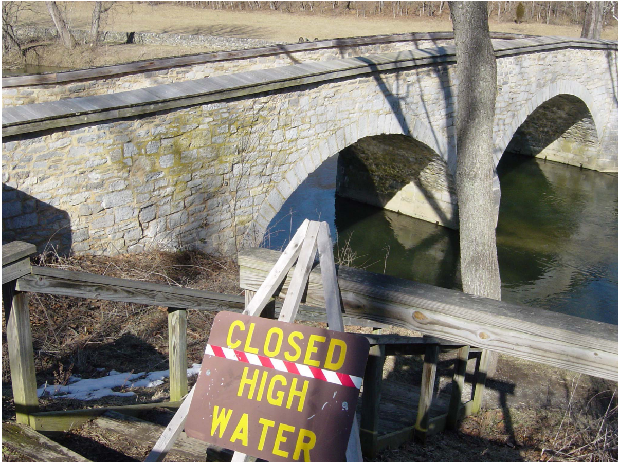
Figure 1: High water damage at Antietam National Battlefield. Erosion from flooding along Antietam Creek disrupts visitor trail access and causes resource management concerns about the protection of Burnside Bridge at Antietam National Battlefield. Photograph by Trista L. Thornberry-Ehrlich (Colorado State University).
