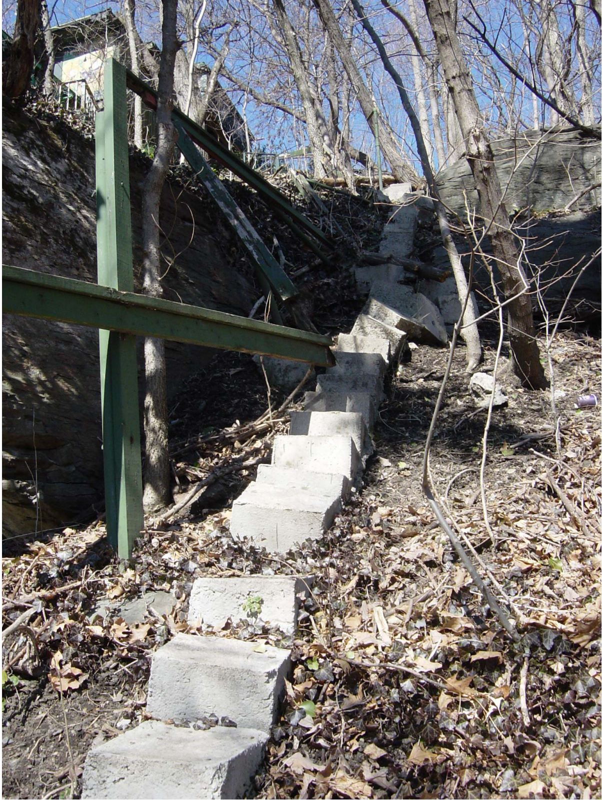
Figure 3: Slope processes at Harpers Ferry. Slope creep and erosional undercutting have undermined this private stairway above Harpers Ferry National Historical Park. Such processes have the potential to destroy trails along slopes and bury features below. Photograph by Trista L. Thornberry-Ehrlich (Colorado State University).
